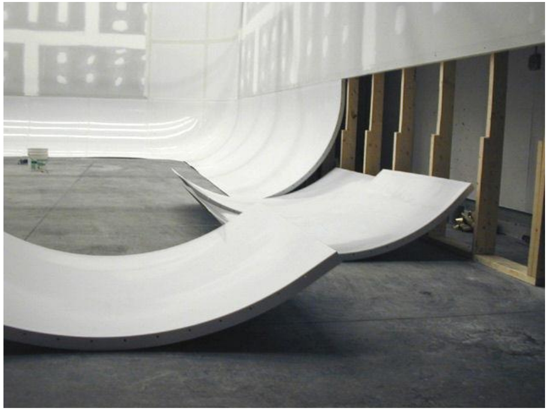
Super 4BI Built-in cove modules install into a false wall built to accommodate cabling and rigging behind the cyc.
